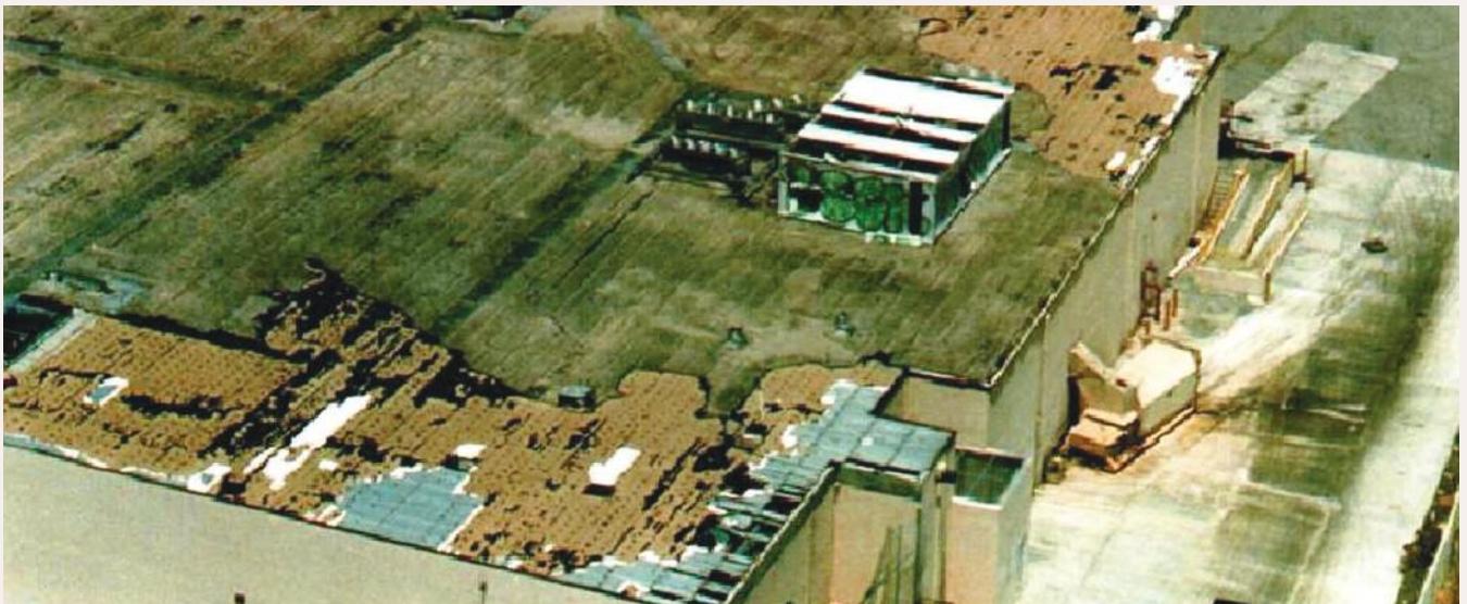
Hurricane damage to this roof is concentrated at the corners and perimeter, where the uplift pressure is higher.
